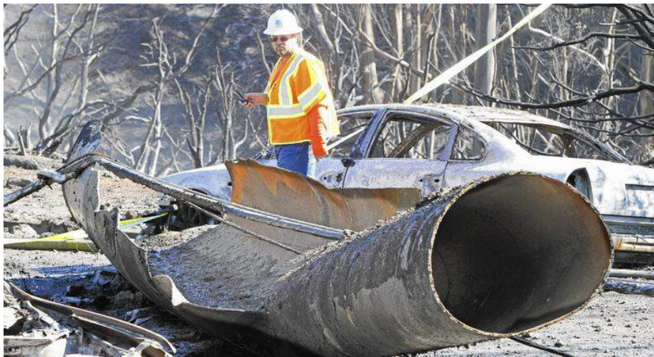
"The morning after the 2010 explosion in San Bruno, a PG&E utility inspector looks at the gas main that ruptured. (Don Bartletti / Los Angeles Times)"
